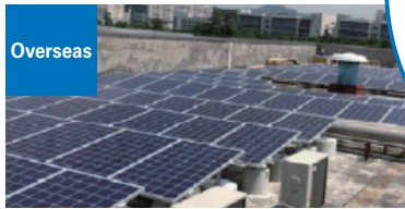
Converted self-generated power to clean energy (Production plant in Guangzhou City, China)
