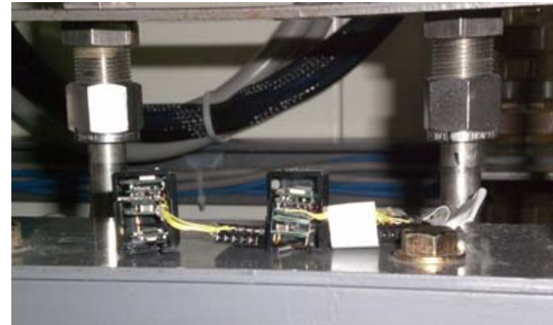
Acoustic & acceleration sensors on a pump
