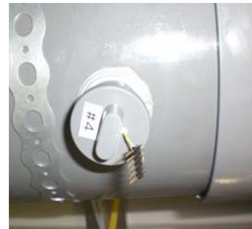
A temperature and relative humidity sensor on an exhaust air duct
