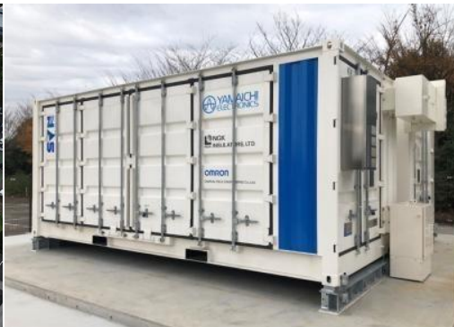
Large-scale storage battery used to secure emergency power source. Battery charged with solar power generated in excess of requirements
