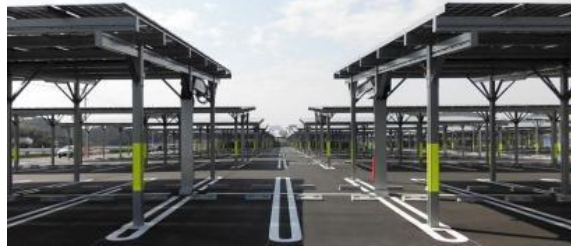
PV power generation systems installed on car port roofs
