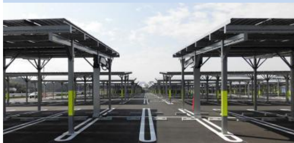
PV power generation systems installed on car port roofs
