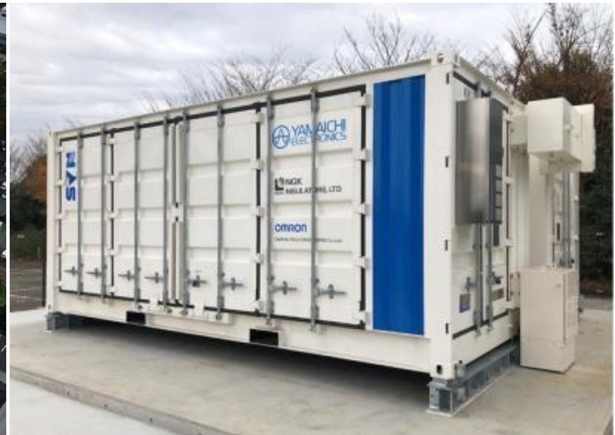
Large-scale storage battery used to secure emergency power source. Battery charged with solar power generated in excess of requirements
