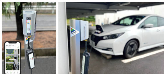
EV charging smart plug module (top) installed in an EV charging outlet to provide an EV charging and billing service
