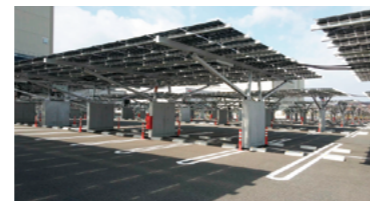
Carport type solar power generation system
