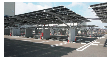
Carport type solar power generation system
