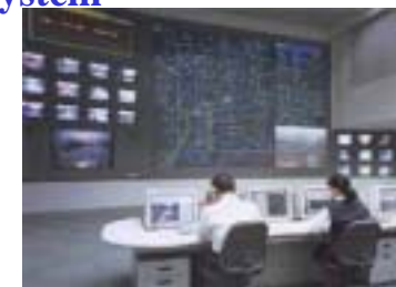
Traffic/Road Management System
